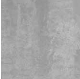
Concrete hell (DP*)
